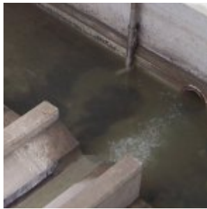
Level measurement using NivuBar Plus in stormwater overflow tank
